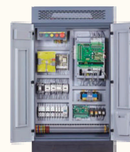
Integrated Lift Controller
